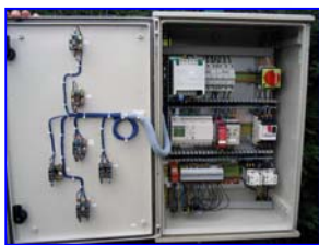
Electrical control panel
